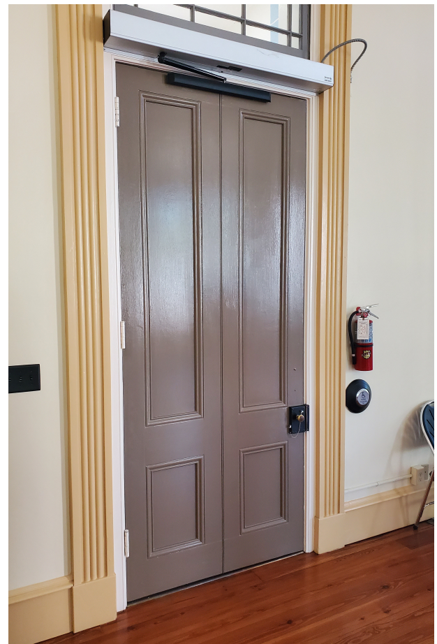
Union Bank of Florida. View of side entrance via exterior handicap ramp, from interior. The image depicts new door that visually resembles original double doors (including restored original hardware) but is a single door meeting width and threshold requirements and has an automatic door opener to meet door opening regulations.
