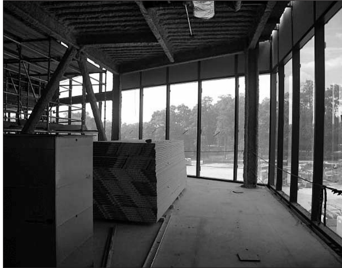
The Siebert Center under construction in the Athenaeum (photo by Linda Barone)
