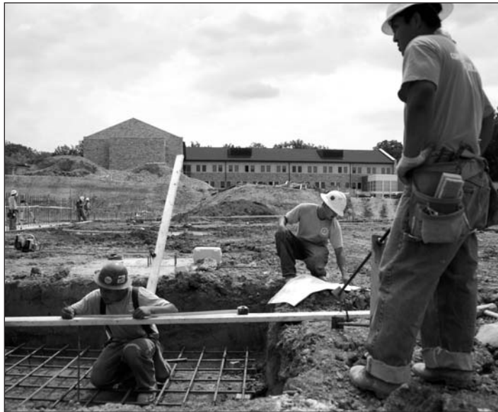
The construction crew begins work on the Athenaeum. Photo by Bob McPeak
